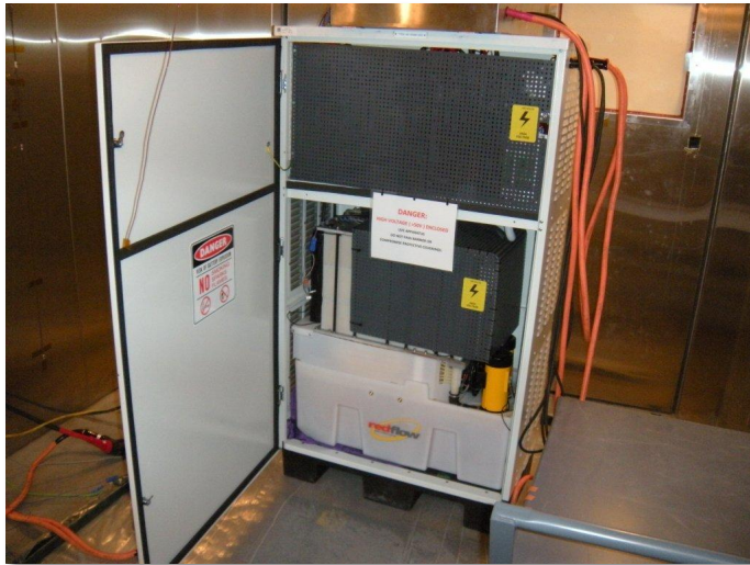
RedFlow SDK Undergoing Temperature Testing
