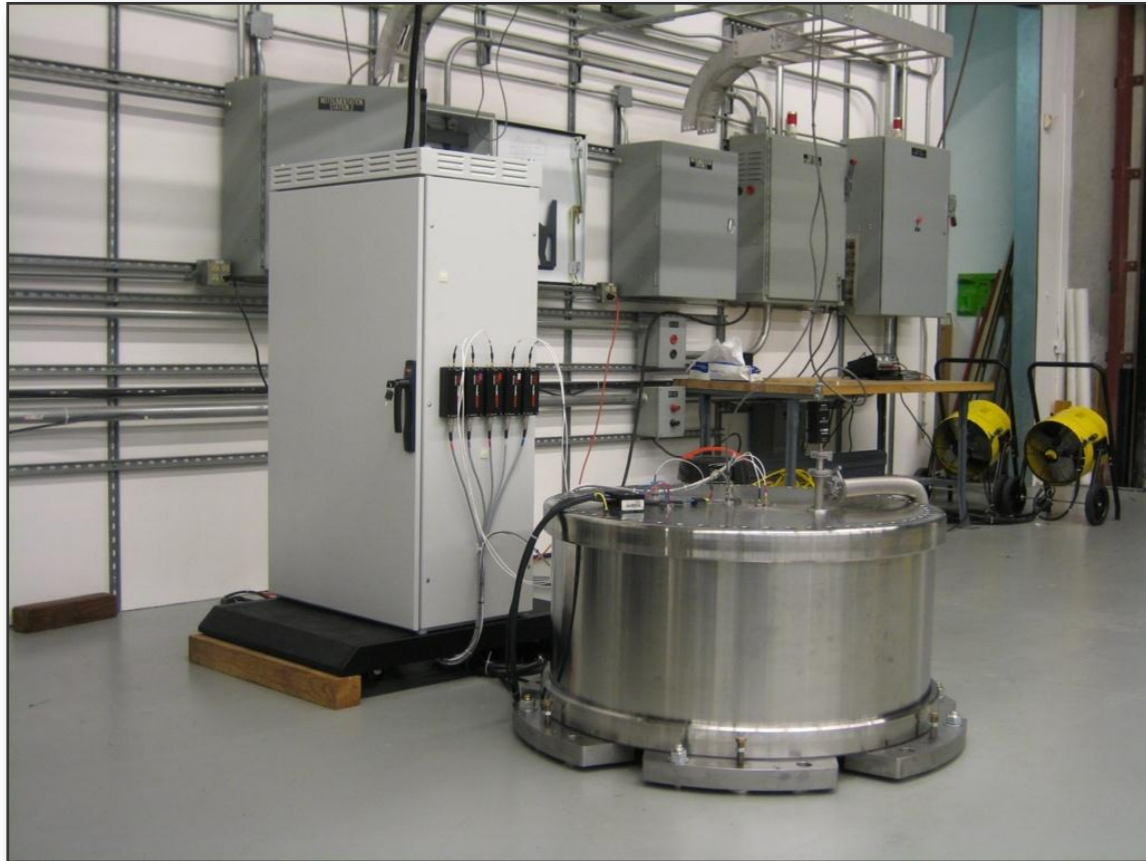
Generation One: Prototype 20 kW | 5 kWh Flywheel System
