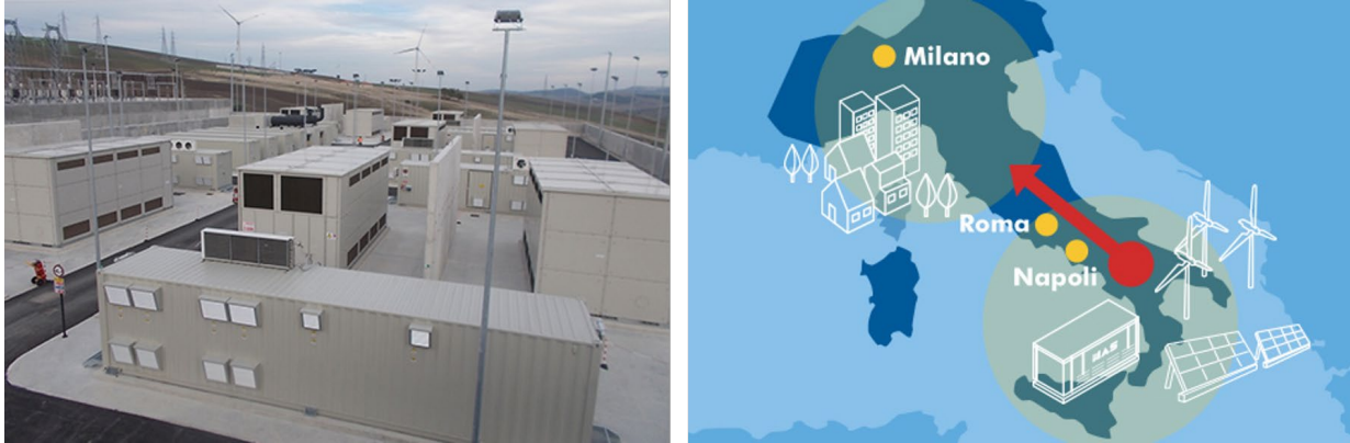
Figure 5. An NAS battery installation in the Campania region of Italy is used to facilitate renewable energy transmission. Images courtesy of NGK Insulators, Ltd. ( https://www.ngk-insulators.com/en/product/nas/ )
