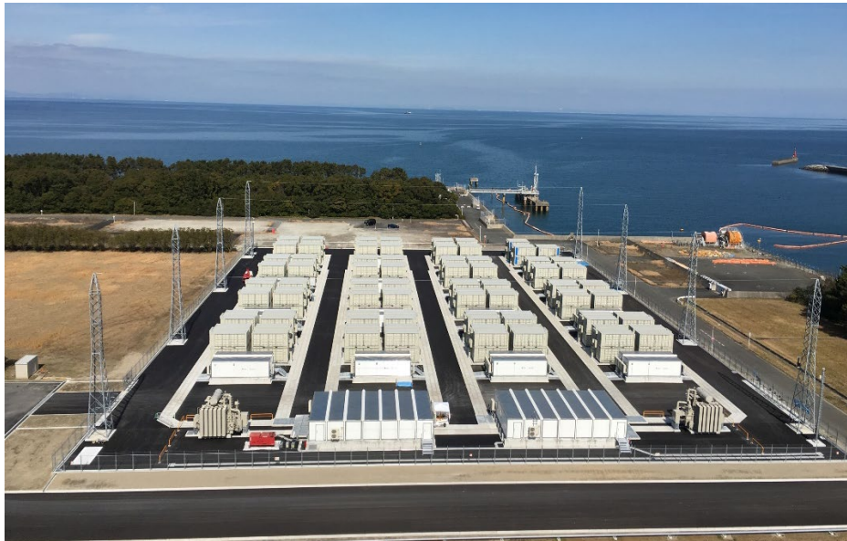
Figure 4. A 50 MW storage system supporting a solar array in Fukuoka, Kyusyu, Japan. Image provided courtesy of NGK Insulators, Ltd. ( https://www.ngk-insulators.com/en/product/nas/solutions/ancillary/index.html )
