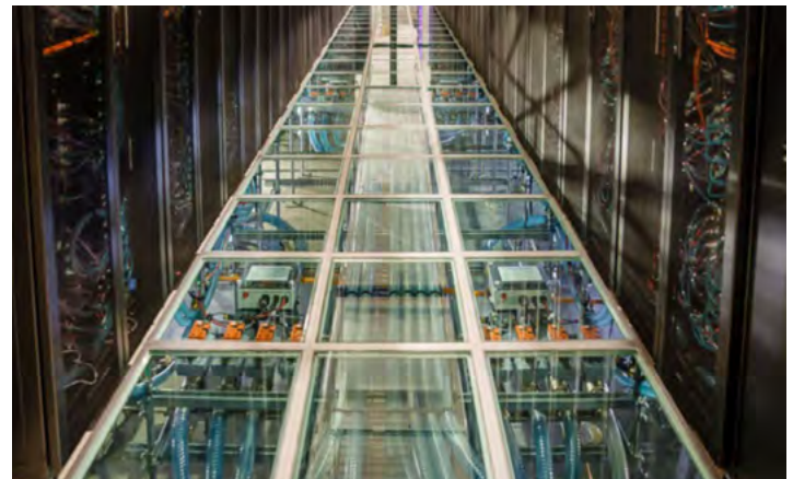
HIGH-PERFORMANCE DESIGN — Building 725E's novel cooling system saves millions of gallons of water annually. Photo by Bret Latter
