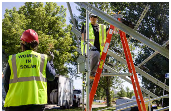
BRIDGING THE GAP — Fifteen Native American women participated in a photovoltaic training installation program at the Red Cloud Renewable Center in Pine Ridge, South Dakota. Sandia’s Sandra Begay provided some of the training as part of a Cooperative Research and Development Agreement.
