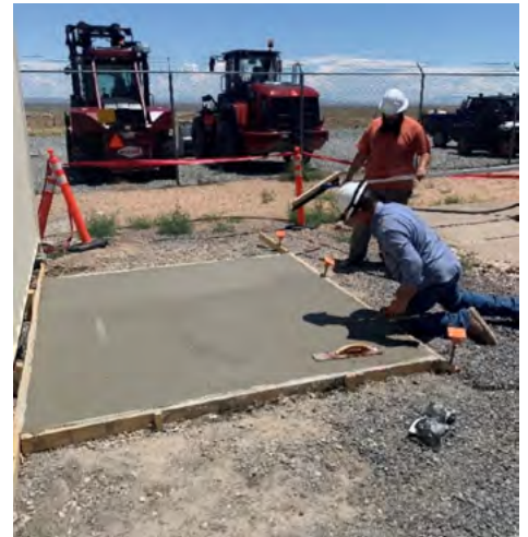
FOUNDATIONAL WORK — Carpenter tradesmen Kevin Pole, in blue, and laborer Fernando Marquez lay concrete. Kevin and Fernando are members of the In-House Construction team.
