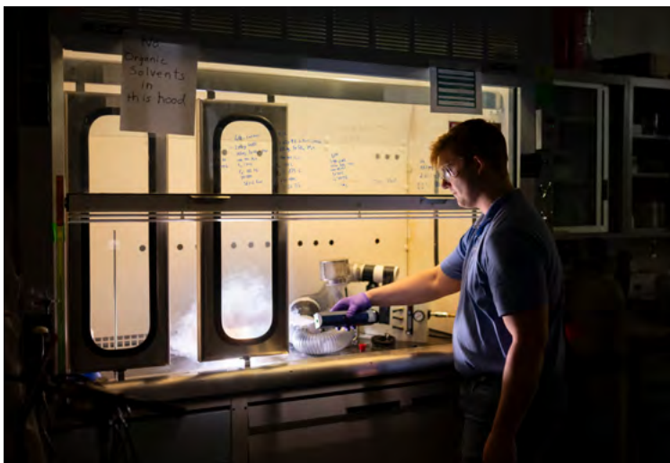
EFFICIENT UPGRADE — As part of the Smart Labs initiative, 3Flow contractor Walker Smith tests fume hoods in building 897 after they are retrofitted to save energy. Photo by Craig Fritz
