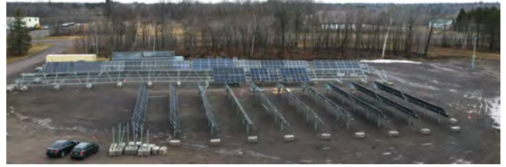
CHANGE IN LATITUDE — Located in the state’s Upper Peninsula, the Michigan Regional Test Center at Michigan Technological University supports Sandia’s research activities on the performance and reliability of photovoltaic systems at northern latitudes. Photo by Paul W. Dice
