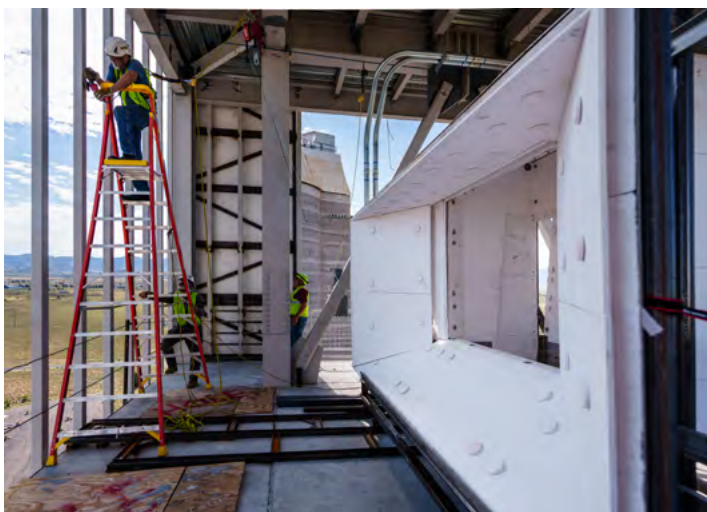
RECEIVER ON DECK — The Generation 3 Particle Pilot Plant receiver sits on rails ready to be moved up to the front of the new tower.
