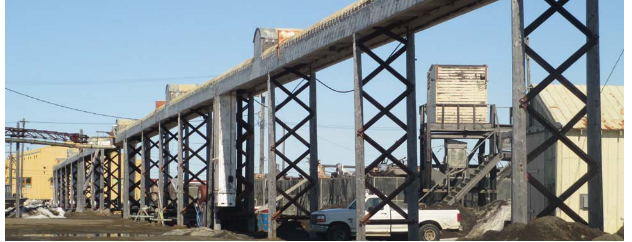
UTILITY CORRIDOR AT BARROW, set high above the ground for the former Naval Arctic Research Lab, now provides service to ARM and other parts of Barrow. Utilities are routed above ground for easy access and are heated in winter. The ground is frozen too solid for winter access to buried lines.
