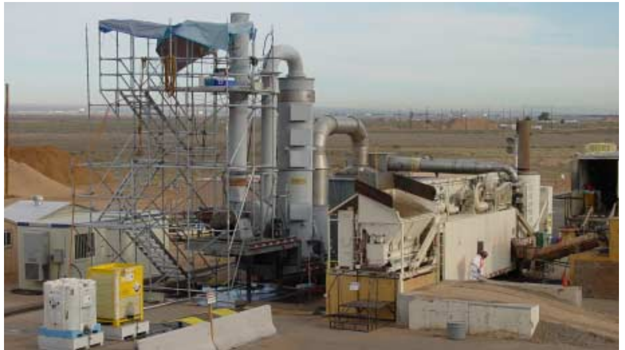
THE KEY TO ON-SITE TREATMENT of chemical waste-contaminated soils from the Chemical Waste Landfill is the Low Temperature Thermal Desorption unit operated for Sandia's CAMU by URS Group Inc. After several years of preparation, the CAMU site at Tech Area 3 was activated last week.
