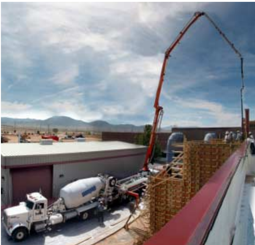
CONSTRUCTION CREW MANAGES a huge 80-yard concrete pour at the east end of Micoelectronics Development Laboratory to form a Specialty Gas Room for the MESA project. The pour was done on Aug. 23.
