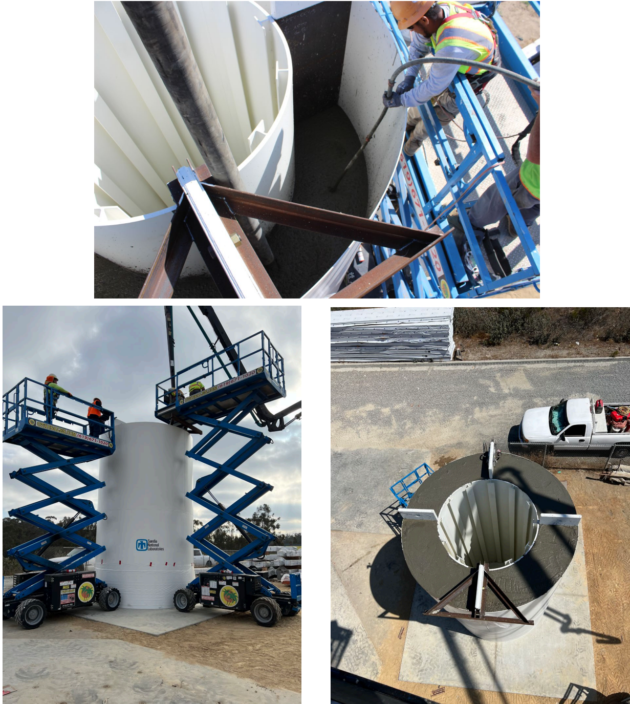
Figure 3-20. Pouring concrete into the cask (top and bottom left) and filled with concrete cask (bottom right).
