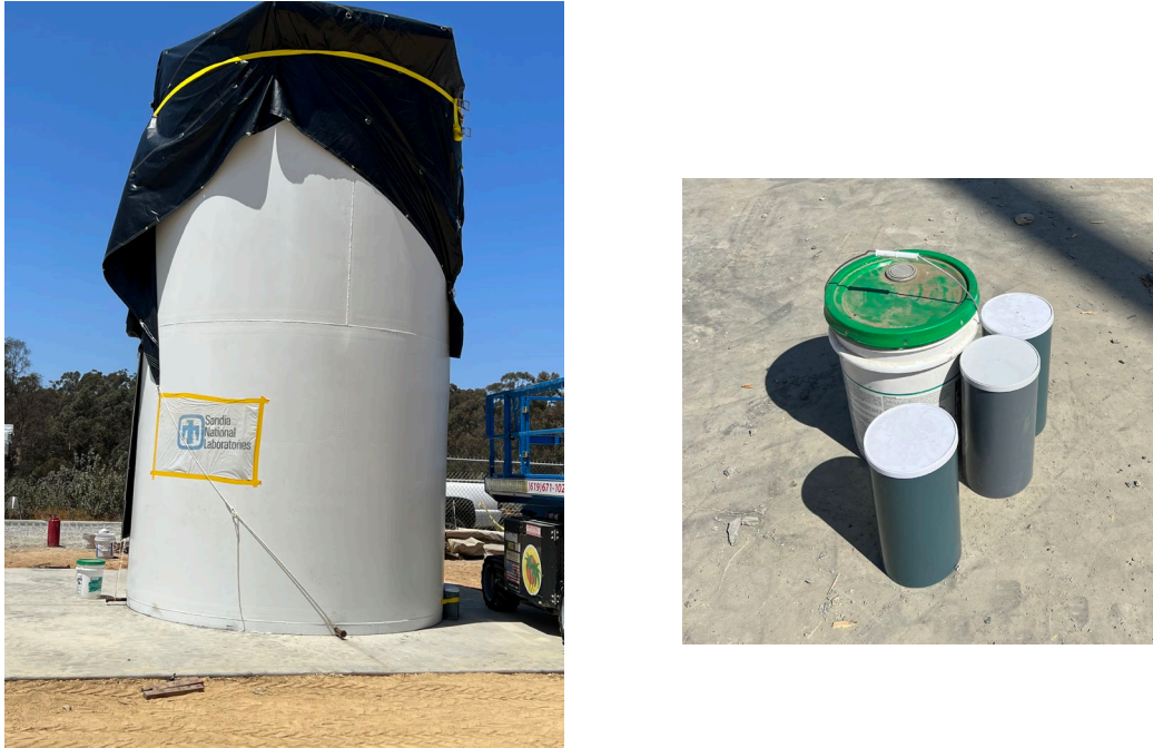
Figure 3-21. Completed vertical cask covered with the tarp (left) and concrete samples (right).
