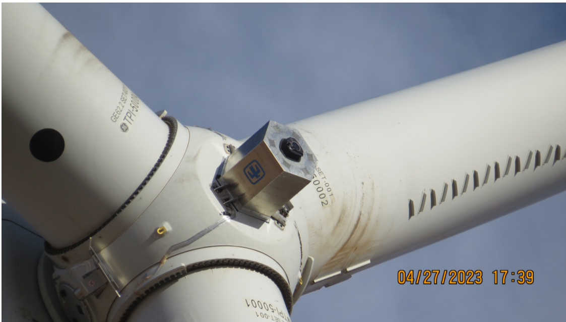
Spinner Lidar installed on the hub of the GE 2.8 MW turbine in Lubbock, Texas and collecting inflow data for the RAAW experiment. (Photo by Tommy Herges)
