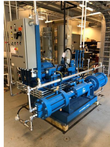
50 kW pilot scale steam generating heat pump
