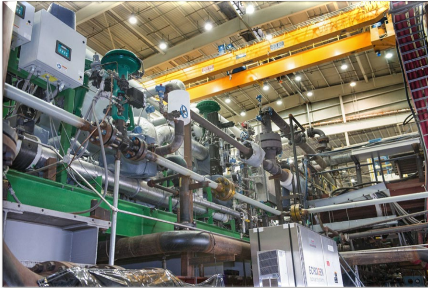
7.3 MW EPS100 during factory test
