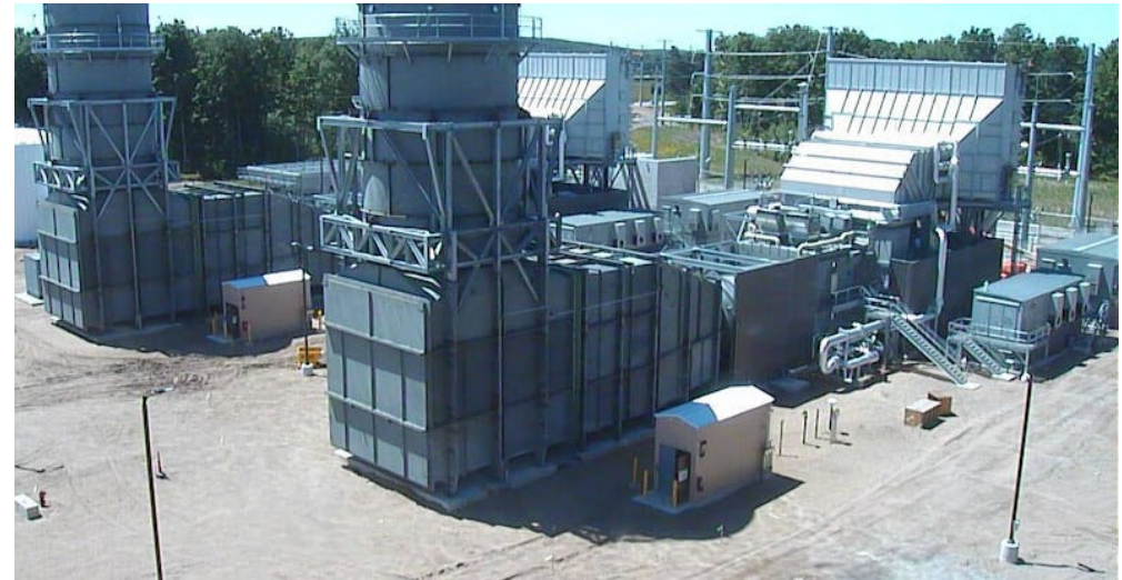
420 MW Simple Cycle Generation Peaker Plant
