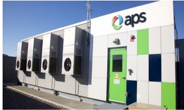
2019 A fire in an ESS in Surprise, AZ leads to an explosion injuring first responders
