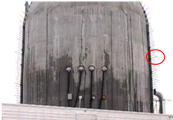
b) Second tendon to rupture, elevation ~ 7.5 m. Approximately 3 seconds before rupture of the containment.
