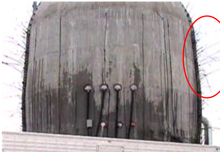
b) Rupture of the containment, major tendon rupture at elevation ~ 5 -10 m.
