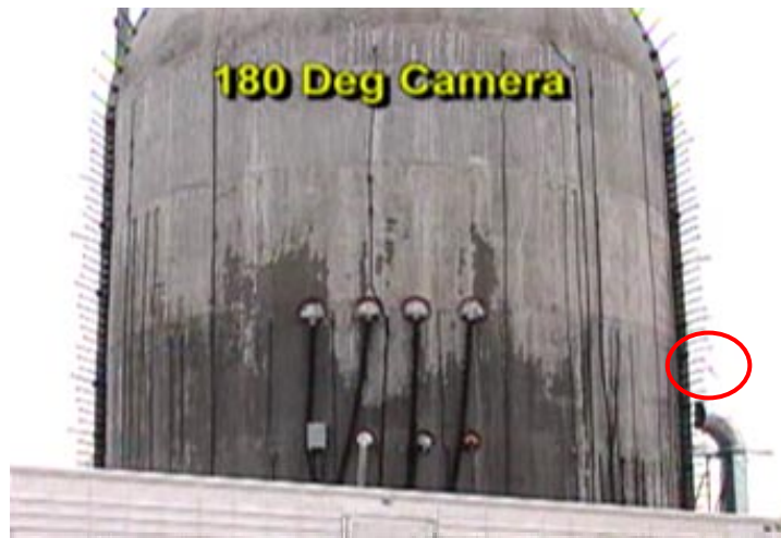
a) First tendon to rupture, elevation ~ 5.0 m. Approximately 15 seconds before rupture of the containment.
