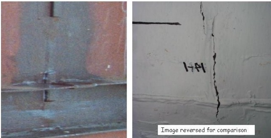
Figure 2. Photographs showing region of tear #1 from outside of liner (left) (prior to concrete placement) and inside of liner (right) (prior to removal of paint). The tear occurred under the wide segment of back-up bar near the top of the left-hand photograph, on the side closest to the anchor.
