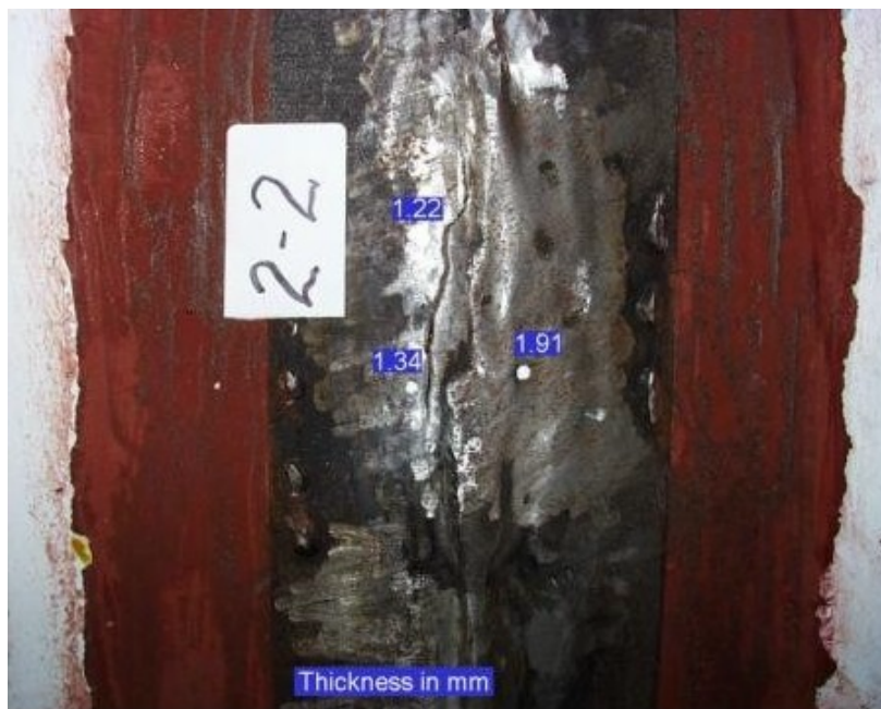
Figure 20. Liner thicknesses (in millimeters) measured ultrasonically in the vicinity of tear #2-2. Note the very wide region of repair welding and grinding. Note also that one measurement is greater than the initial plate thickness due to previous weld repairs.
