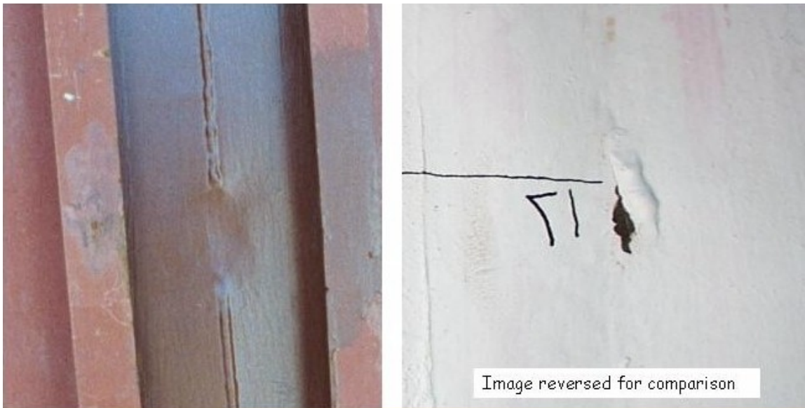
Figure 12. Photographs showing region of tear #17 from outside of liner (left) (prior to concrete placement) and inside of liner (right) (prior to removal of paint). Note how weld bead is ground off on outside surface in vicinity of repair weld (made from inside of liner) and tear.
