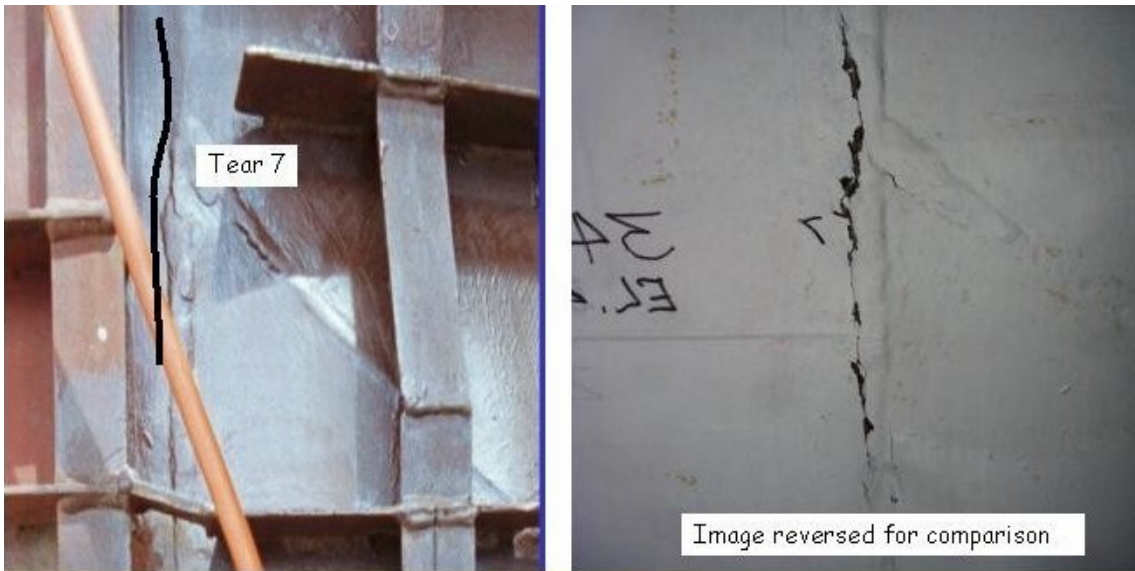
Figure 15. Photographs showing region of tear #7 from outside of liner (left) (prior to concrete placement) and inside of liner (right) (prior to removal of paint).
