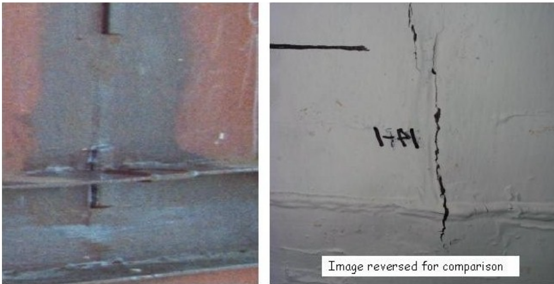
Figure 10. Photographs showing region of tear #14-1 from outside of liner (left) (prior to concrete placement) and inside of liner (right) (prior to removal of paint). Note missing segments of back-up bar in vicinity of repair weld and tear.
