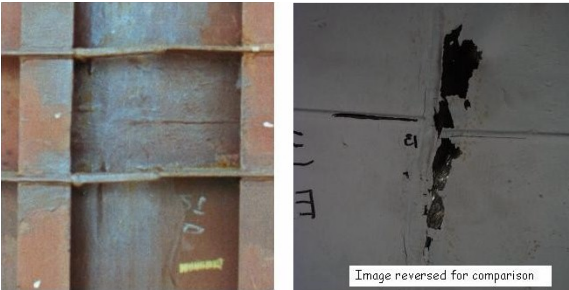
Figure 18. Photographs showing region of tear #13 from outside of liner (left) (prior to concrete placement) and inside of liner (right) (prior to removal of paint).
