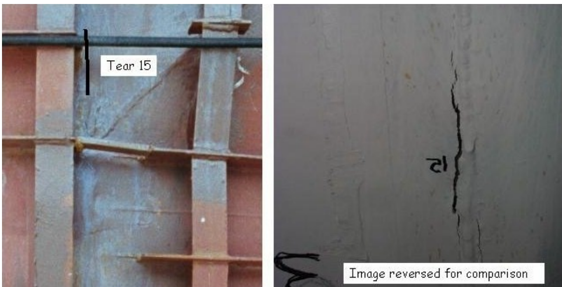
Figure 16. Photographs showing region of tear #15 from outside of liner (left) (prior to concrete placement) and inside of liner (right) (prior to removal of paint).
