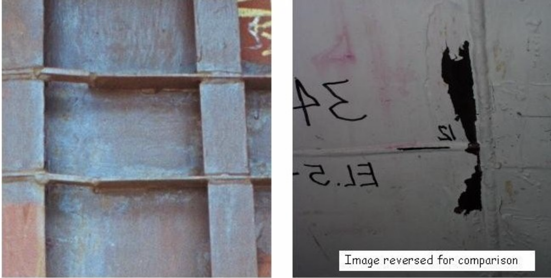
Figure 17. Photographs showing region of tear #12 from outside of liner (left) (prior to concrete placement) and inside of liner (right) (prior to removal of paint).
