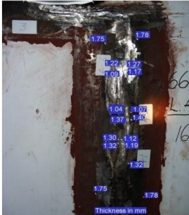
Figure 21. Liner thicknesses (in millimeters) measured ultrasonically in the vicinity of tear #4 (4-1, 4-2, and 4-3).
