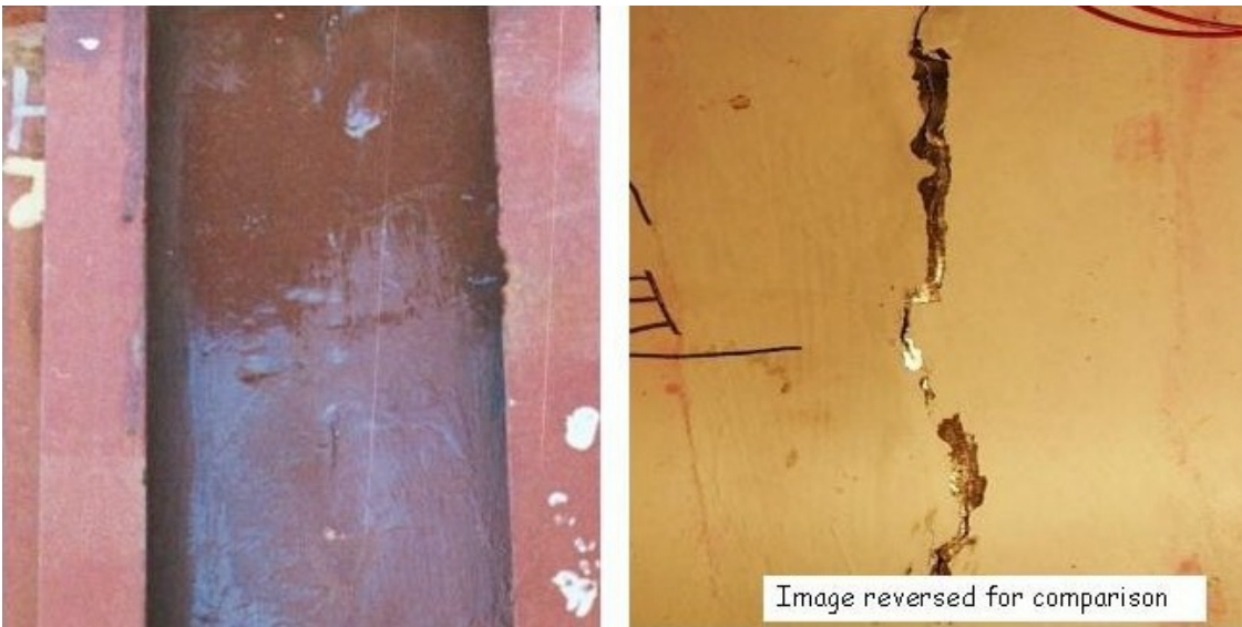
Figure 4. Photographs showing region of tear #4-1 from outside of liner (left) (prior to concrete placement) and inside of liner (right) (prior to removal of paint). Separate tears began of opposite sides of the weld, eventually growing together through the fusion zone.
