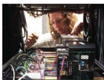
Chantel Nowlen inspects rod control rack power supplies.
