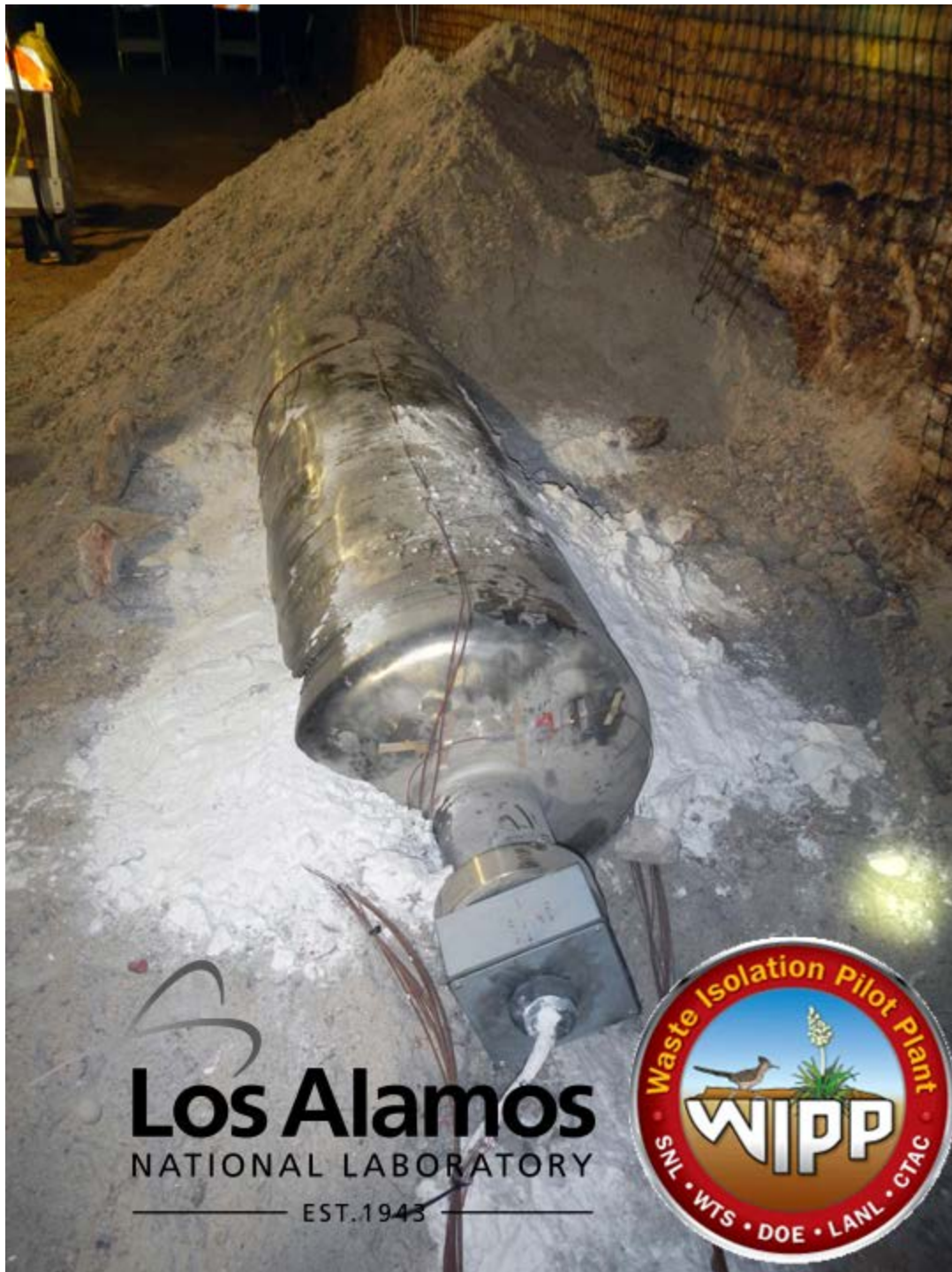
Figure 50: End view of intermediate stage of salt placement. For this experiment, cuttings from rockbolt holes (bright white salt) are applied to protect wiring and thermocouples (exposed wiring).
