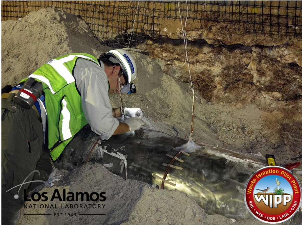
Figure 51: Installation of vertical thermocouple arrays extending from top of can towards top of pile.
