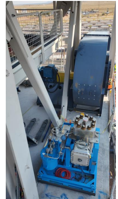
sCO 2 blower (heat rejection) (top) and sCO 2 pump (bottom)
